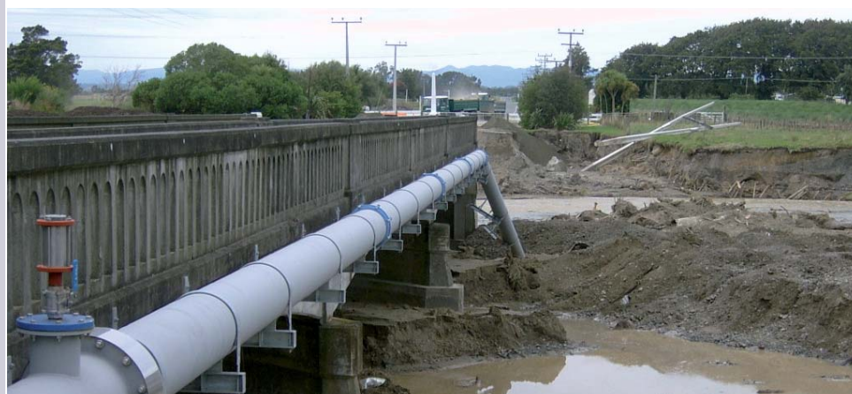
Fielding Bridge after the 2004 flood gives a dramatic image of interdependency between utilities
