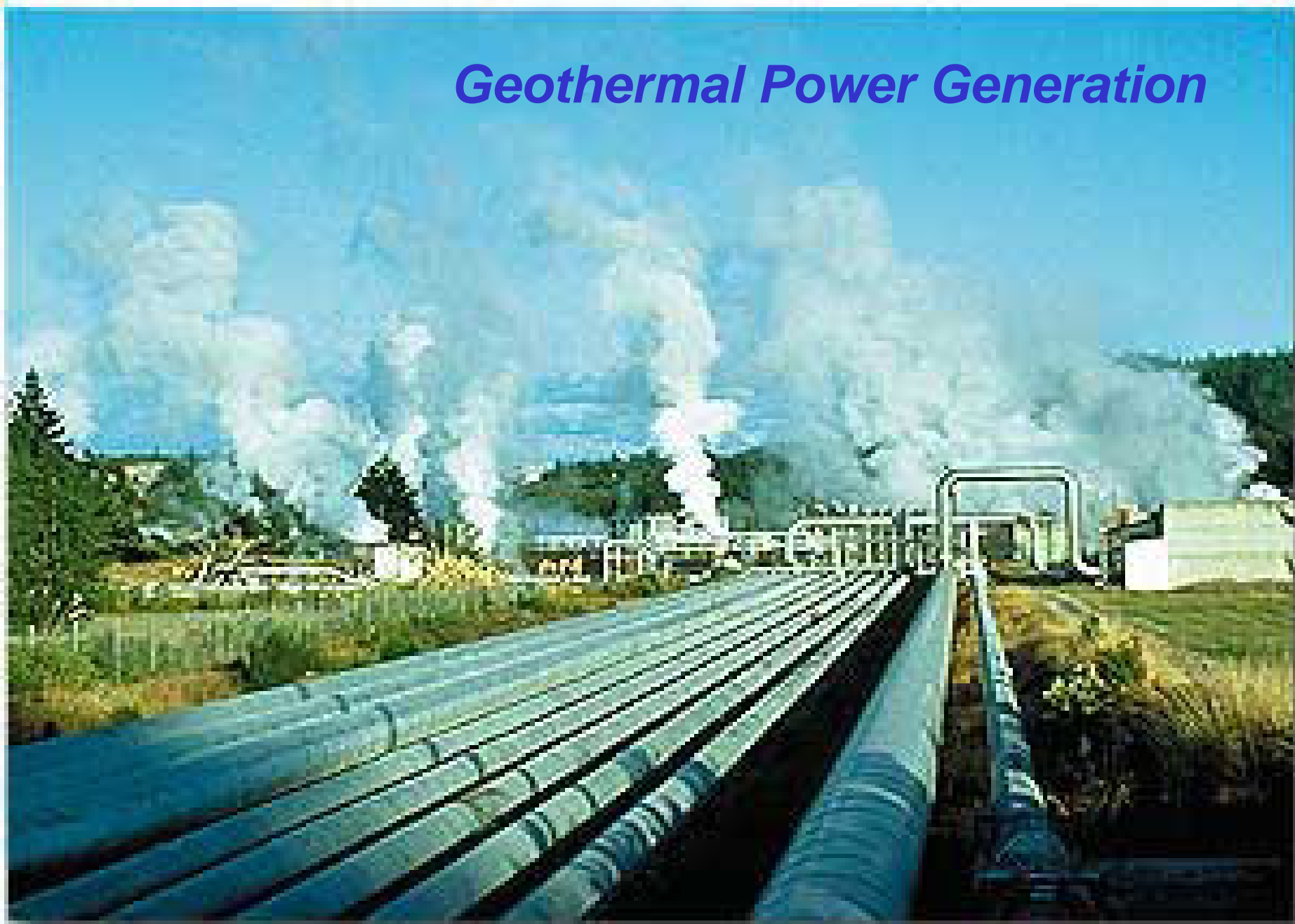
Steam pipelines, Wairakei Power Station
